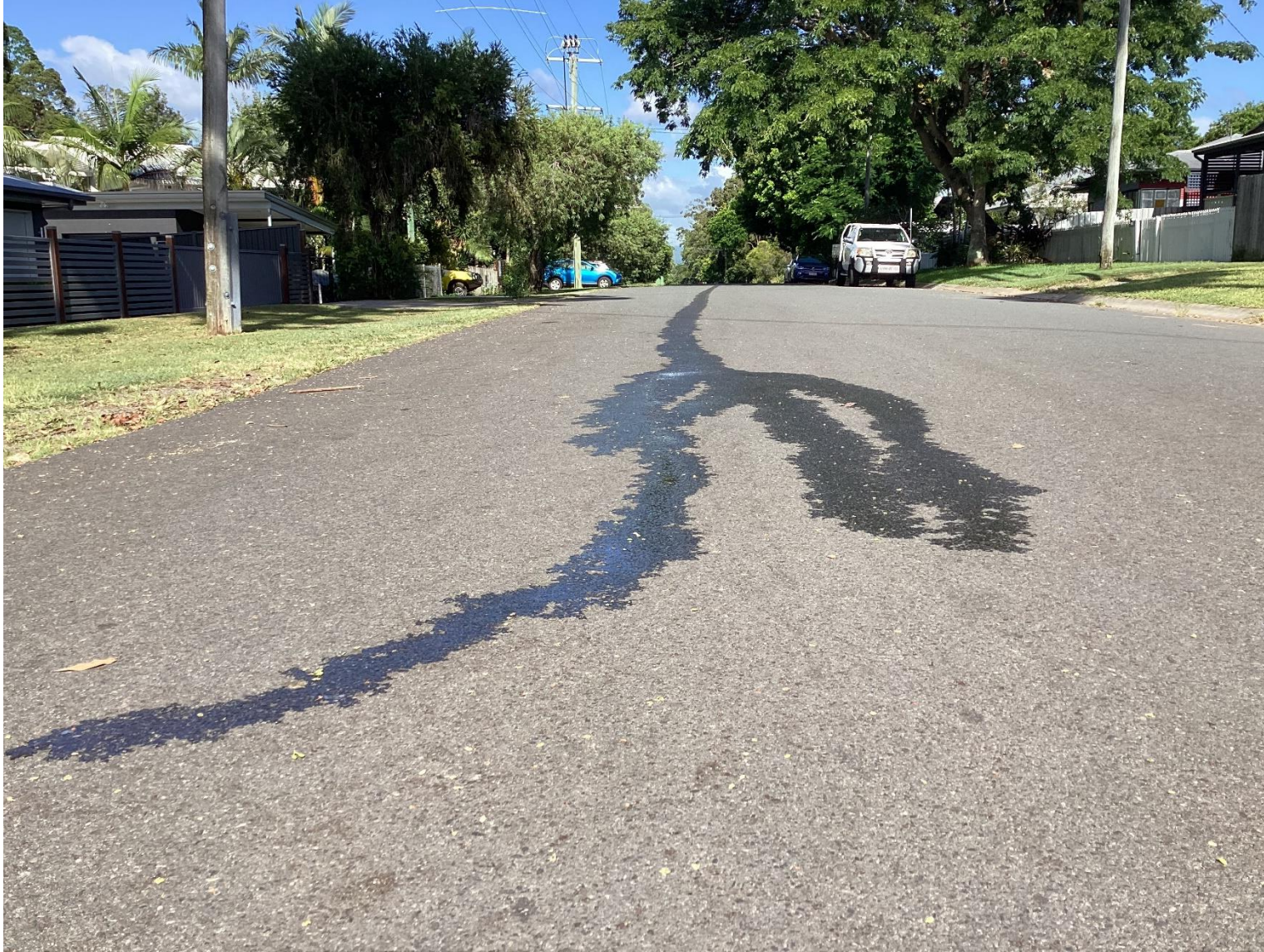
Figure 1. Van wastewater on Laguna St
